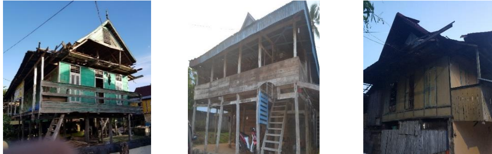
Figure 1. The wrecked Buginese Bone Aristocratic traditional house abandoned by its dwellers Source: Survey photograph, 2020
